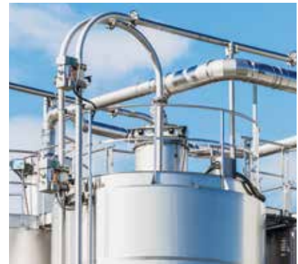
Silos within a chemical plant
